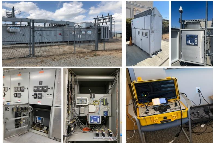
Fig. 2. Examples of real-world WMU installations in Riverside, California: (left): 3-phase 12.47 kV installation at a substation; (top-right): 3-phase 480 V installation at a PV inverter; (bottom-right): single-phase 120 V installation at a power outlet.
